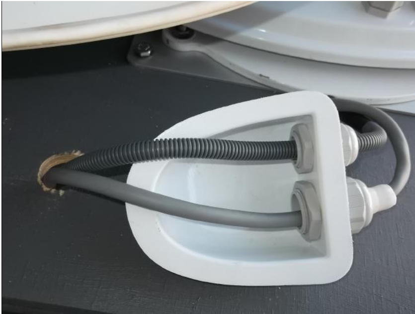
Junction Box with the loom from the dome entering a 1” hole into vehicle.
